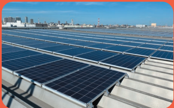
L's Power Station Toda Bijogi (Owned by LOTTE Financial Corporation)
